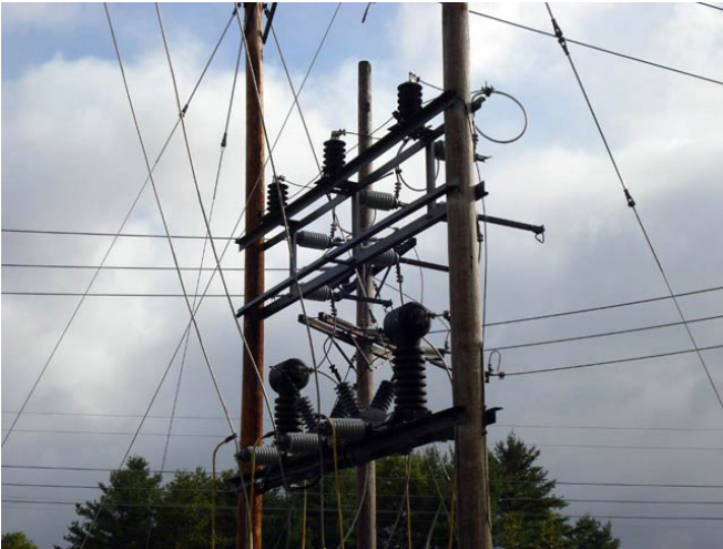
Above: Pattenville Station Source: Littleton Water and Light
