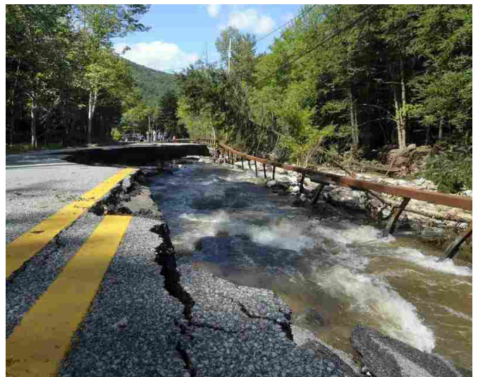
Above: Road damage from Hurricane Irene. Source: National Public Radio
